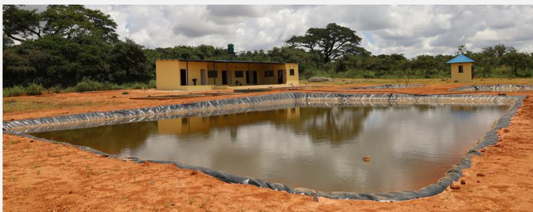
Figure 1 Pond based system using dam liners (Source: WorldFish Center/NRDC, 2019)
