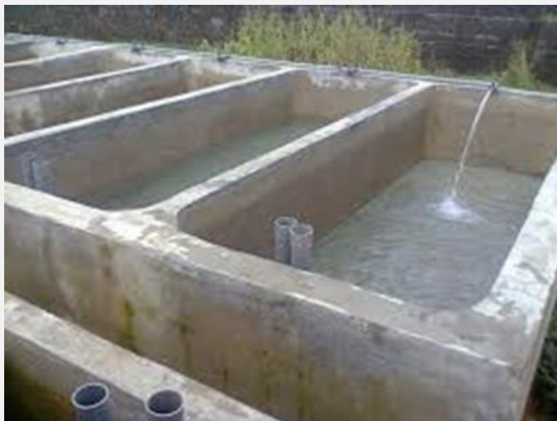
Figure 8 Stagnant Concrete Tank in North Central, Nigeria
